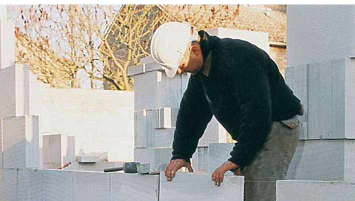
Faster build times and increased productivity on site are offered with the thin joint system, particularly when used with Aircrete's large format blocks.
